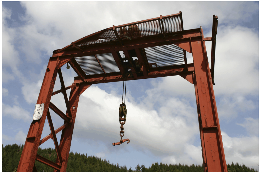
Figure 4-1. Overhead traveling crane.
