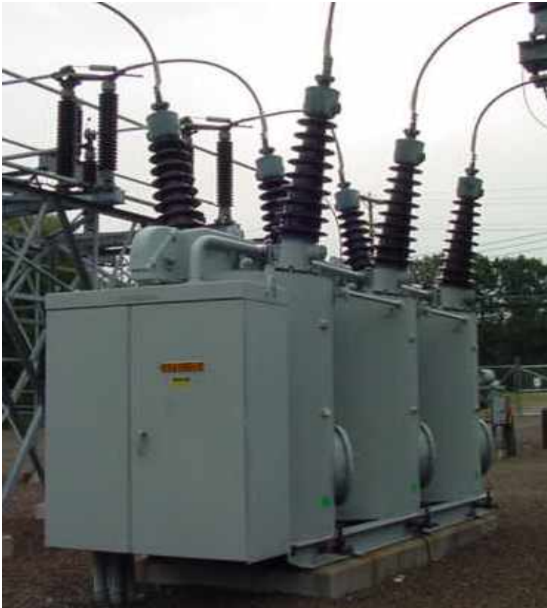
115KV Oil breaker
